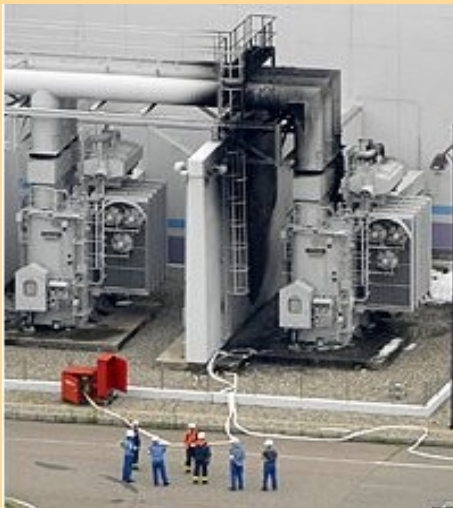
Radioactive material leaked from the Kashiwazaki nuclear power plant
